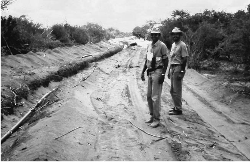
FIGURE 5.1. Grading roadbed and laying out water pipes at Hagadera, Dadaab, Kenya, 1992. (Photograph by Per Iwansson)
