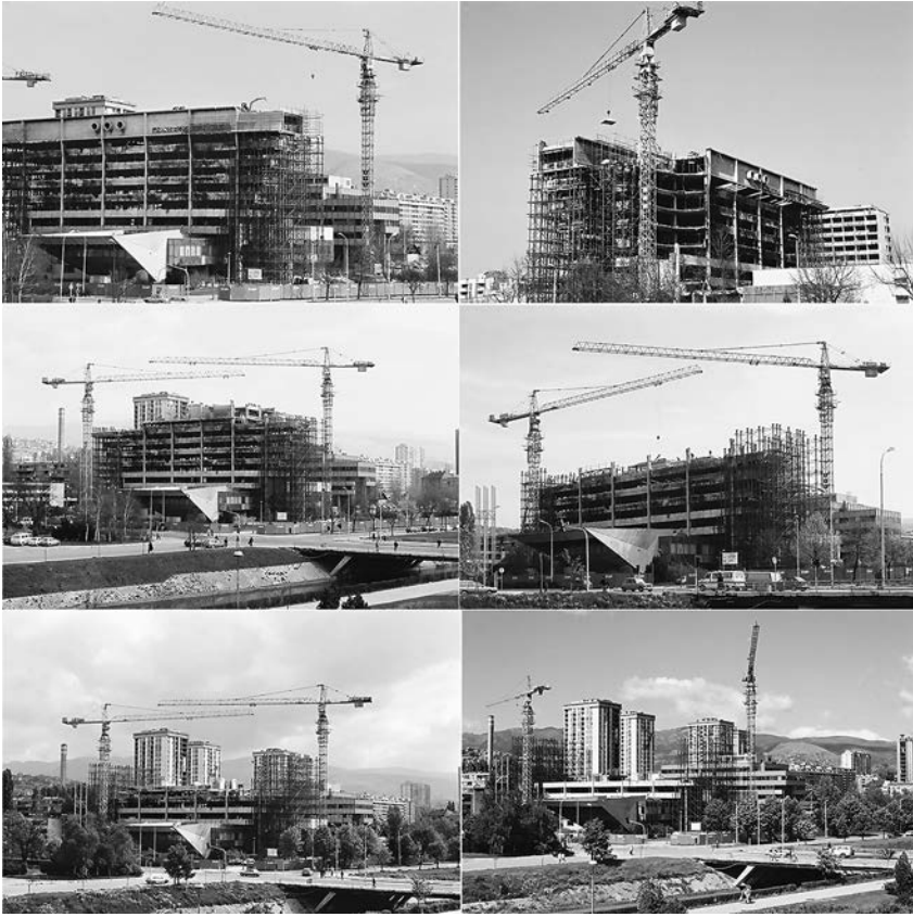
FIGURE 2.7. Composition by the author of the photos showing the cleaning of the ruined parts of the Elektroprivreda Building. (Photograph by Zoran Kanlić, 2000)
